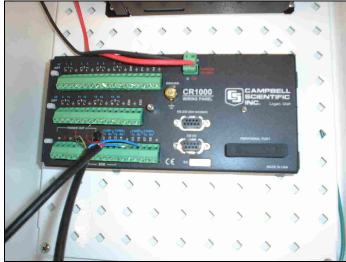
Figure 57: Solar panel connection in to the datalogger
